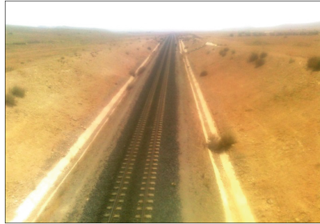
Fig. 3. Filling of drainage channels by sediment
